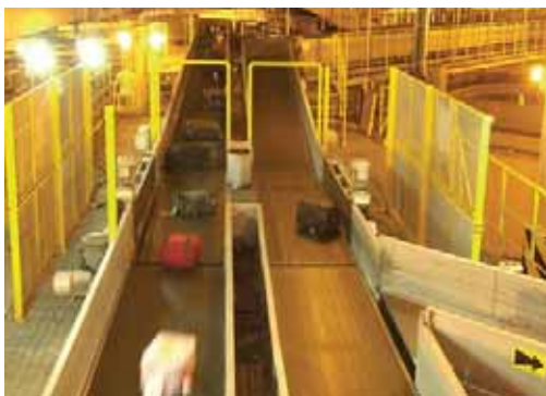
Automated Baggage Handling System
